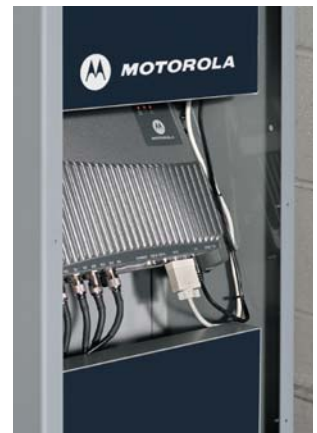
Open view of the portal reveals the fixed reader and antennas in the protective casing.
